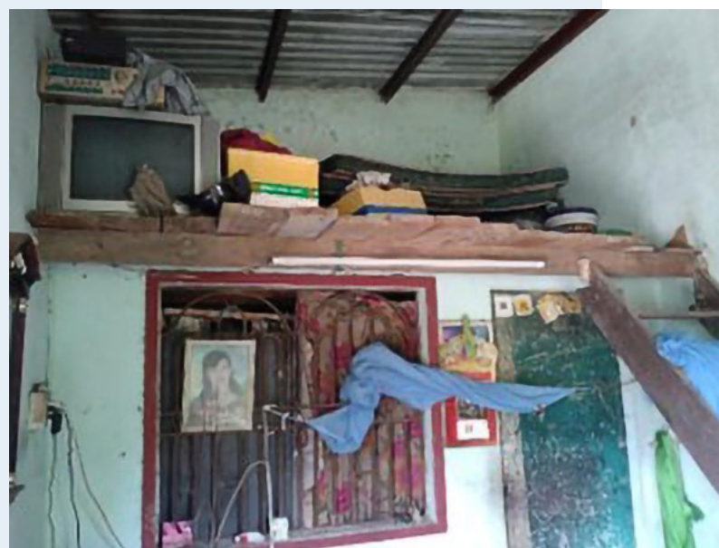
Top photo: Water depth in Mr. Vo's house during the 2020 floods
