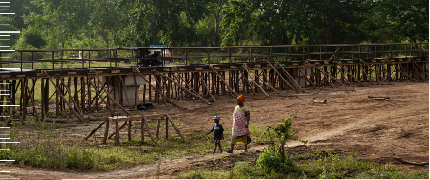
A bridge under construction in Mikameni village in Kenya's Tana River County © Lisa Murray, Concern Worldwide
